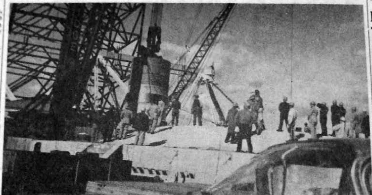
THE WORLD'S LARGEST BEARING is shown above as it was being installed recently at the Naval Radio Research Station in Pendleton
